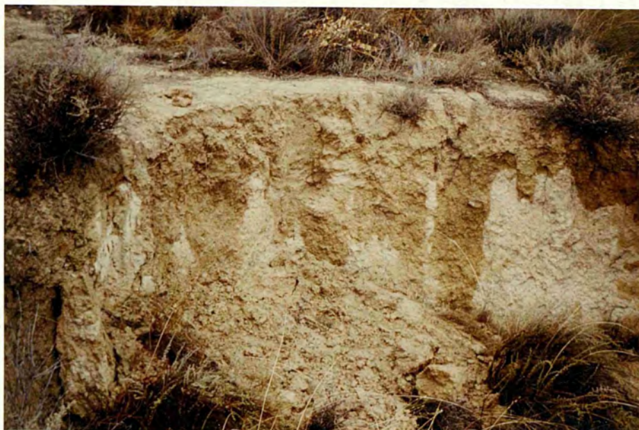
Photograph 7.1 Surface wash over the gully face on site 1
